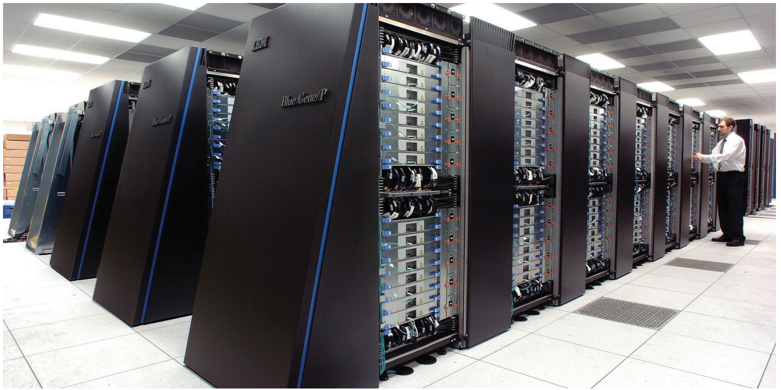
Shown in this 2007 photo is the IBM Blue Gene/P supercomputer installation at Argonne National Laboratory in Lemont, Illinois. (Photo courtesy Argonne National Laboratory)
